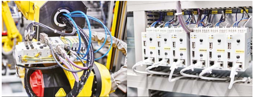
□ Valves with IIoT integration (left), connected to the smart pneumatic monitoring “hubs” (right) aggregate and organize pneumatic performance data and deliver it through separate, parallel pathways to plant management systems.
