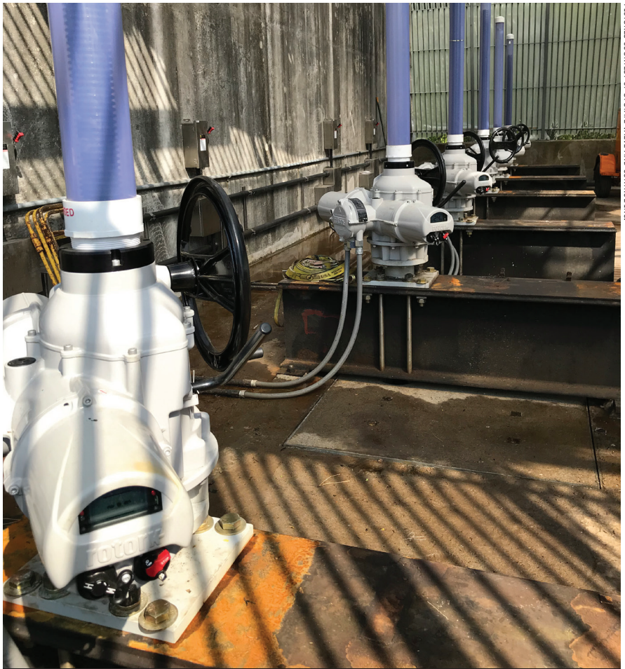
Figure 1. Equipment retrofitted to replace old hydraulic units with new electric actuators
