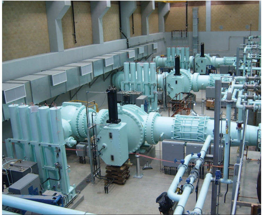
42-inch rotary cone valves and metal-seated ball valves are used in a raw water pumping station, San Vicente, CA.
