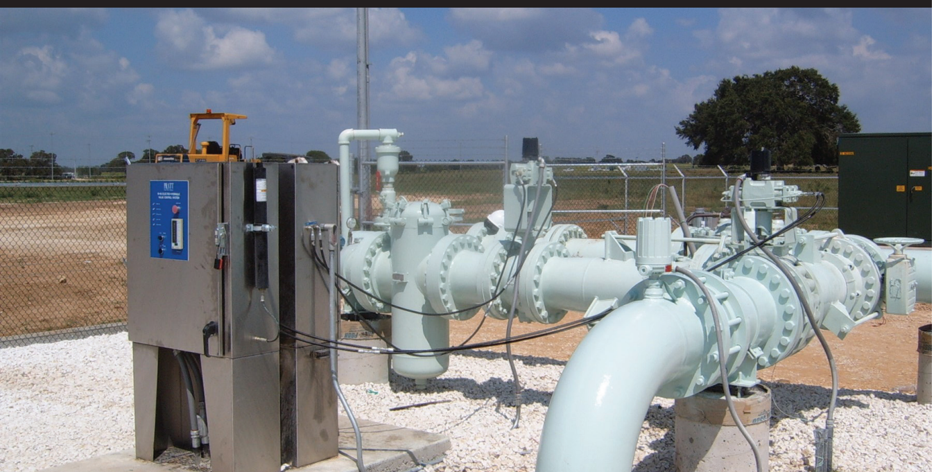
High-pressure hydraulic units control 10-inch and 12-inch high-performance ball valves in an aquifer recharging application, San Antonio, TX.
