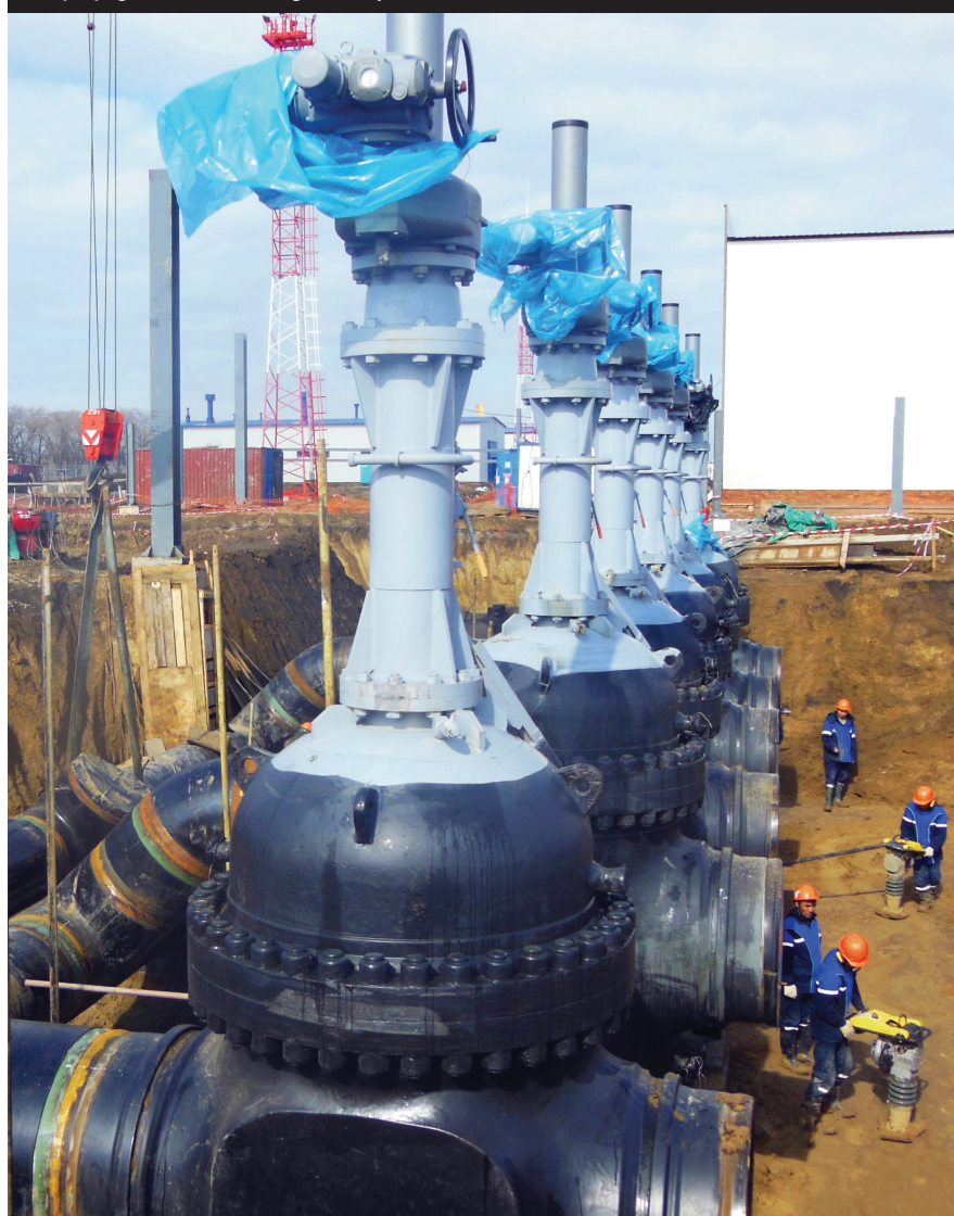
□ A pumping station in the oil and gas industry
