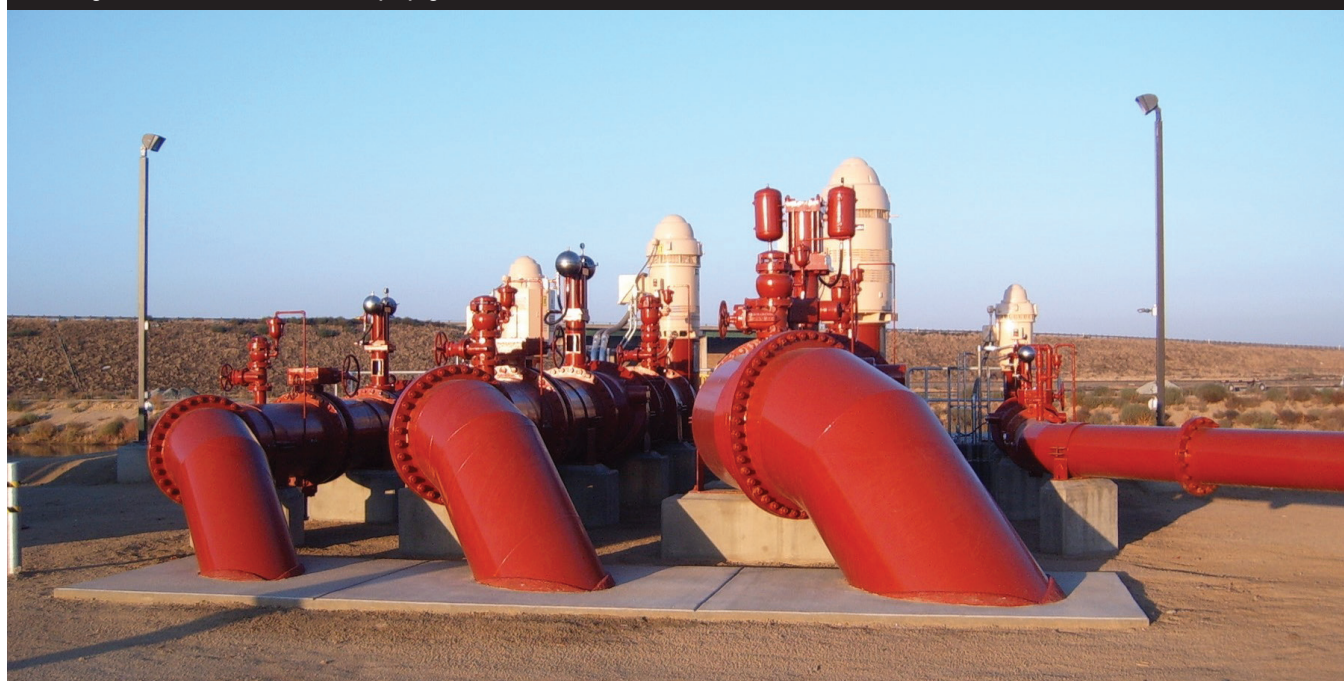
A tilting disc check valve is used at a raw water pumping station in Bakersfield, CA.
