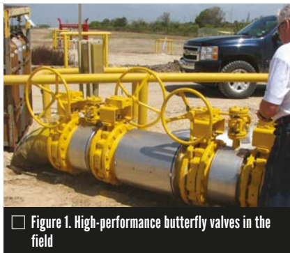
Figure 1. High-performance butterfly valves in the field. The wet chlorine is dried using concentrated sulfuric acid ( H_2SO_4 ). Lined ball or plug valves are often
