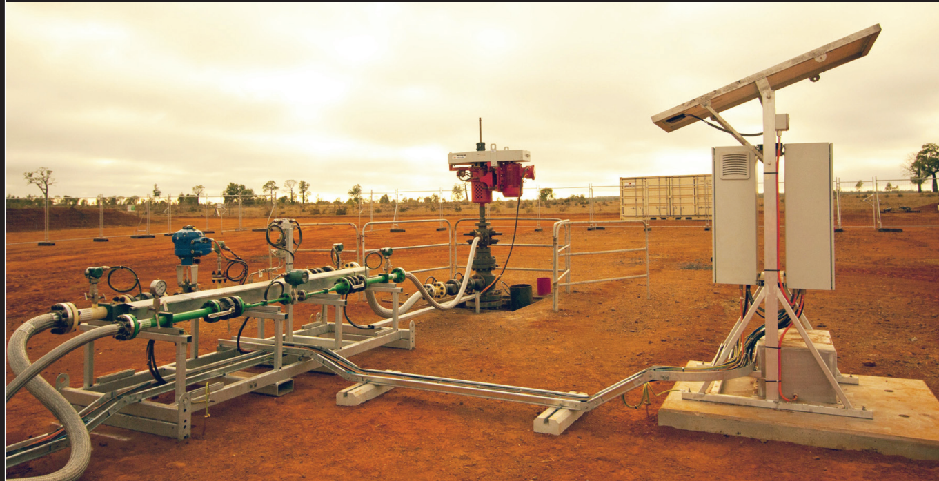
□ This typical oil and gas upstream application using a solar panel powers a failsafe electric control valve actuator.
