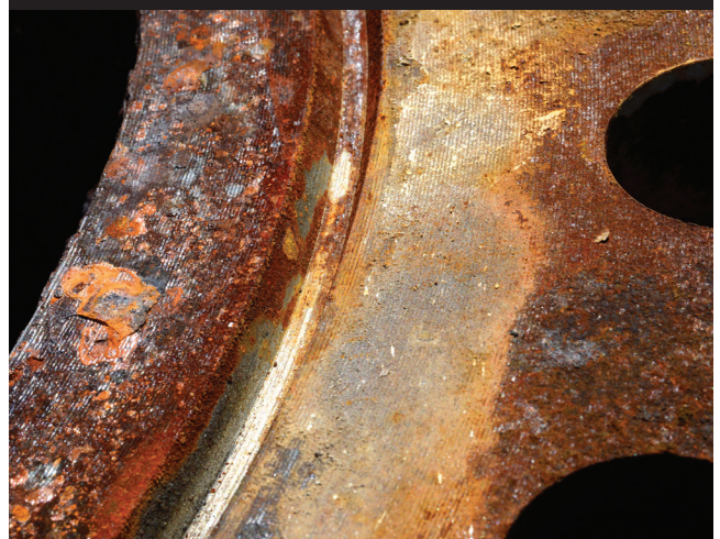
□ RTJ grooves must be smooth on the sides where the gasket touches or leakage will occur. This damaged RTJ groove will require machining and possibly weld repair.
