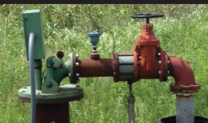
Figure 1. Air release valve on golf course pumping system
