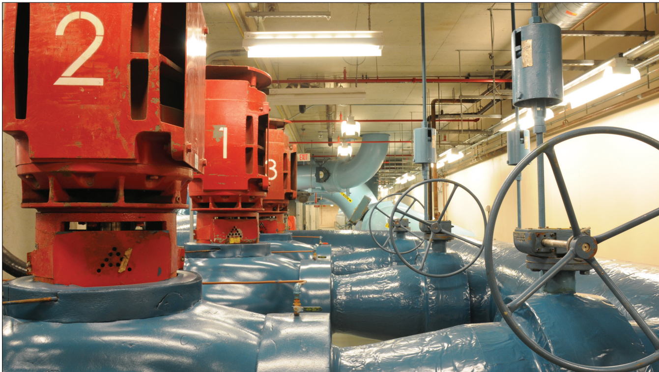
□ Energy transfer station pipe gallery
