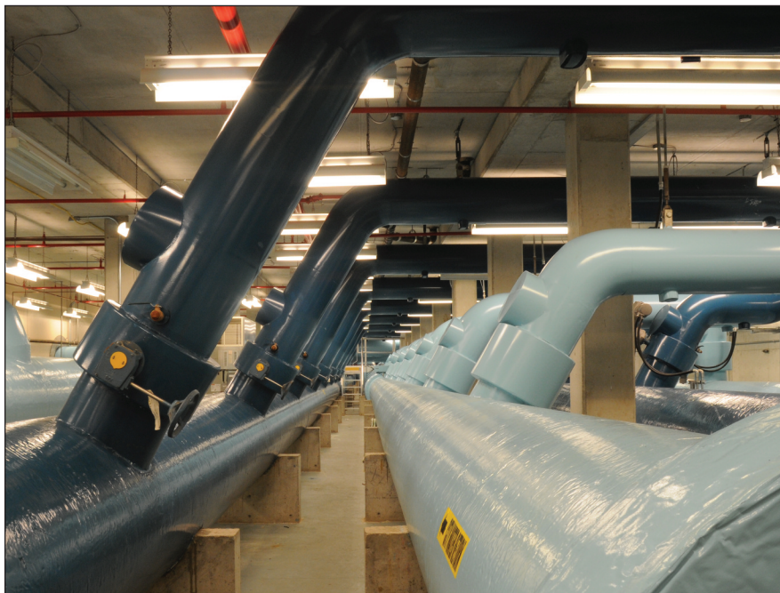
□ Energy transfer station pipe gallery risers to heat exchangers
