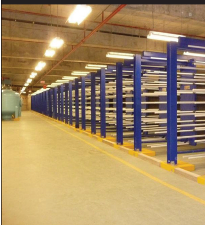
□ Heat exchangers, which provide the way for energy transfer between the cold lake water and the closed chilled-water supply loop
