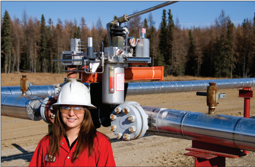
□ Figure 3. 6D application on a flow line equipped for ESD/PSD
