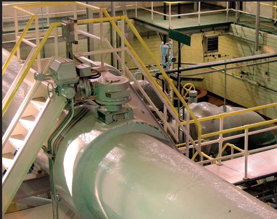
□ A 72-inch butterfly valve regulates water intake from Lake Michigan in one of the Chicago's water purification plants.
