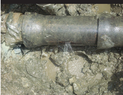
□ The nation's water infrastructure is feeling its age and the lack of sufficient funding.
