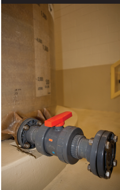
□ Figure 3. A flanged ball valve attached to a tank
