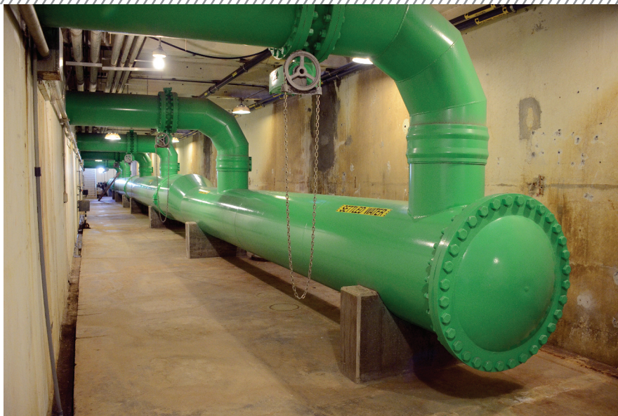
□ These outlet lines from the final sedimentation tanks are made of carbon steel and are equipped with ductile iron butterfly valves.
