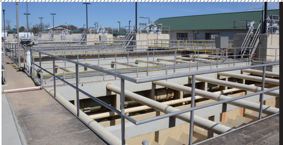
□ The filtration tanks at a typical water purification facility show how numerous valves interconnect each tank and allow each separate unit to be drained for maintenance purposes.
