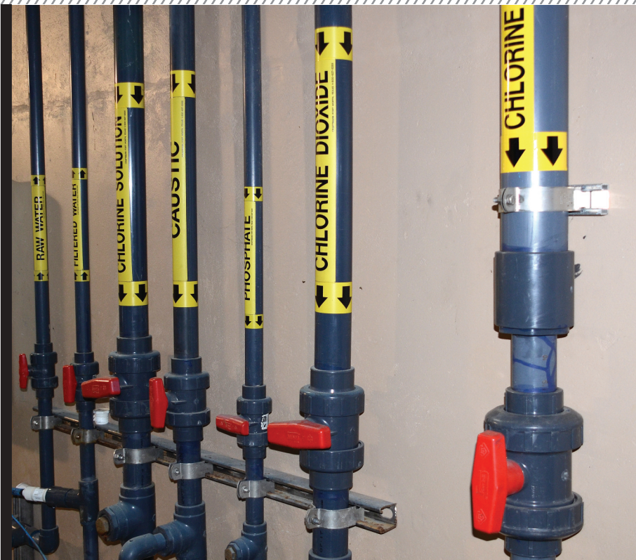
□ These additive and sampling lines are low pressure and are constructed of PVC material, including the ball valves.
