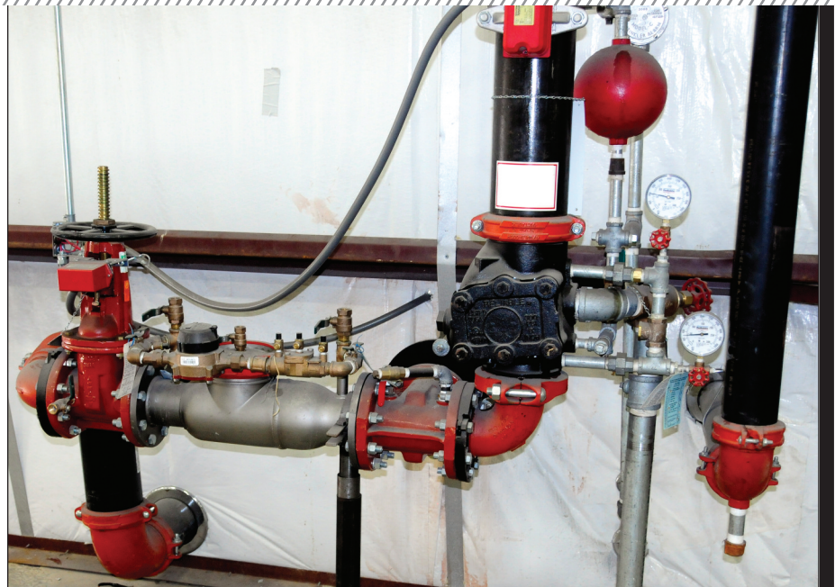
□ In this typical sprinkler system valve installation in an industrial building, the piping includes iron and bronze, gate, globe and check valves. The main isolation valve is interlocked with the fire-alarm system and is activated when the valve is opened.
