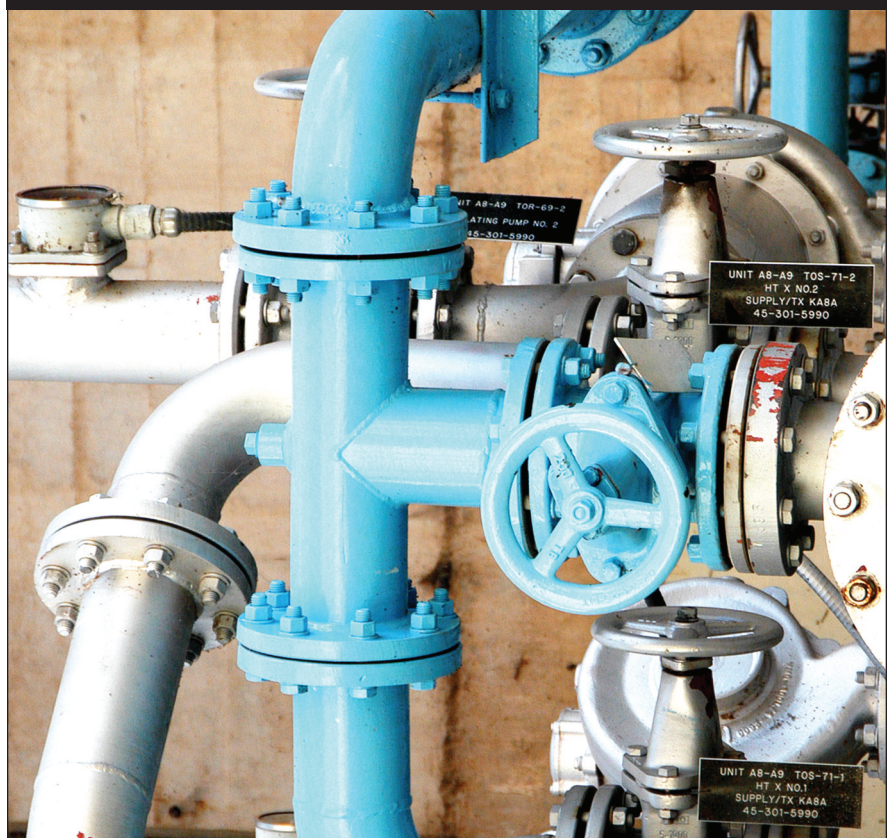
Chiller systems for HVAC applications often contain many valves. This image shows part of the piping system on an industrial chilled water system.
